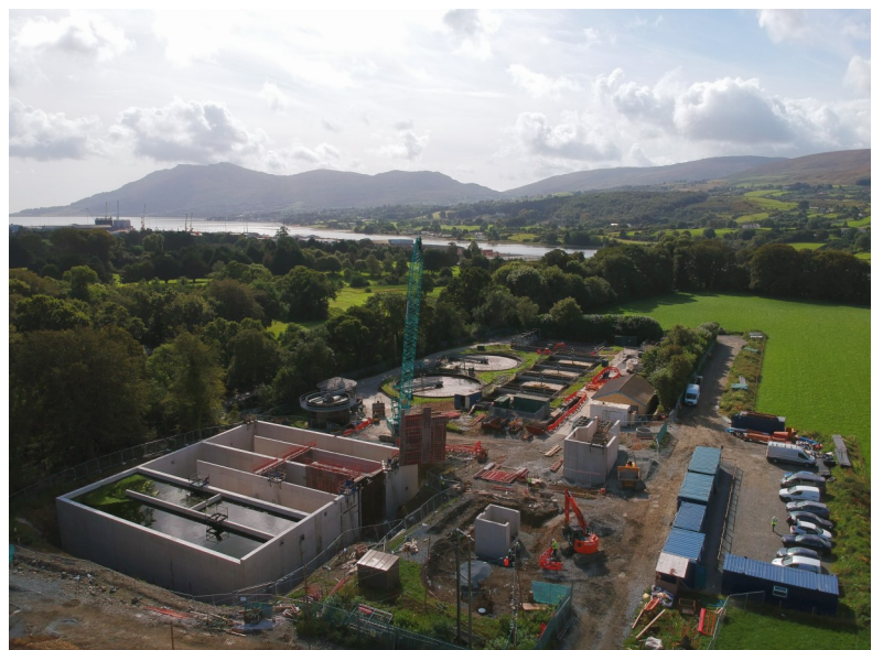
Warrenpoint Waste Water Treatment Works
