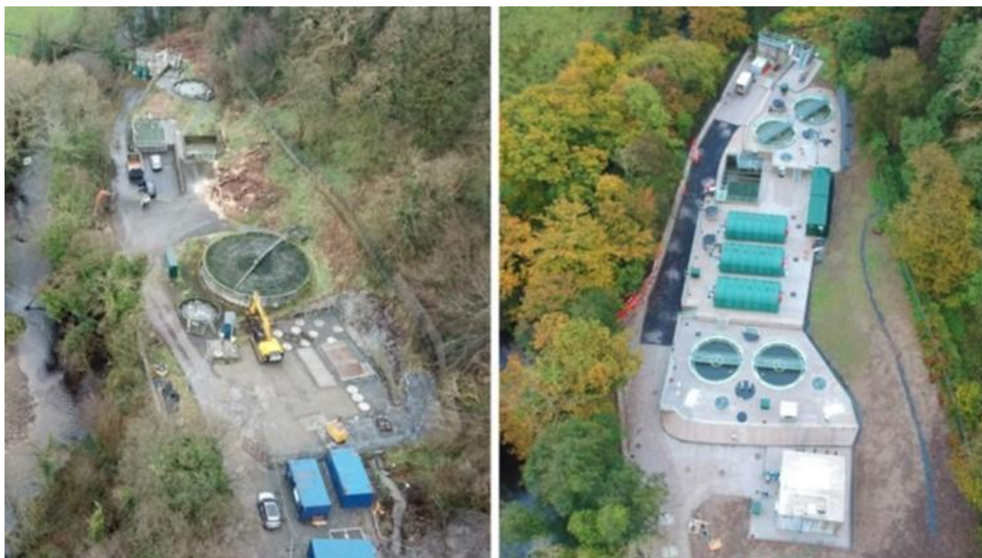
Figure 9.1: Works at the start of construction (left) and the completed Donemana WwTW (right)
